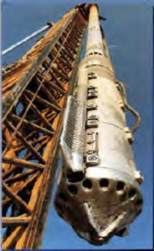
Vibro compaction improved the bearing capacity of the loose, sandy soils and mitigated liquefaction potential for construction
